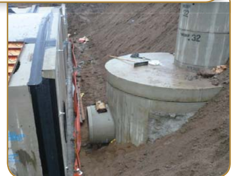
The design allows large rainfall events to bypass the system to prevent resuspension of retained pollutants.
