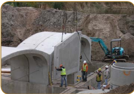
A precast design was used for the system's walls to facilitate the construction schedule.
