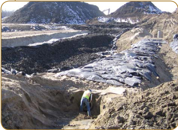
A lightweight fill which utilized a combination of wood chips and shredded tires was used.
