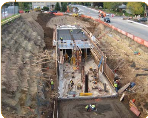
The contractor used stepped slopes to provide safe working conditions in the trench during construction.
