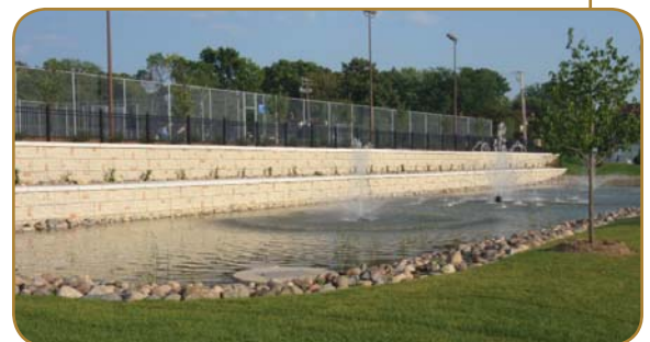
The underground reservoir was custom designed to fit into the available space and was constructed in two phases to accommodate storage of material on the small site.
